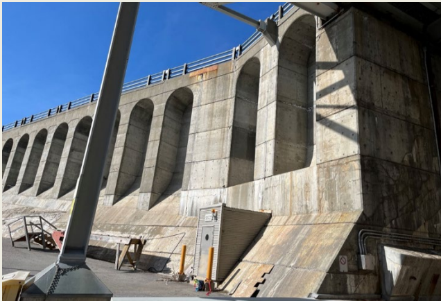
Figure 2b: Section of a dam affected by ASR (Photo credit: Matthieu Argouges, Civil Engineer, Hydro Quebec)
