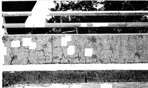
Figure 1b: Cracks observed in 1986 (Photo credit: ICAAR 1986)
